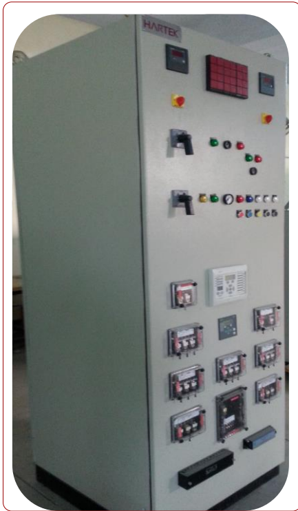
Transformer & Feeder Panel
