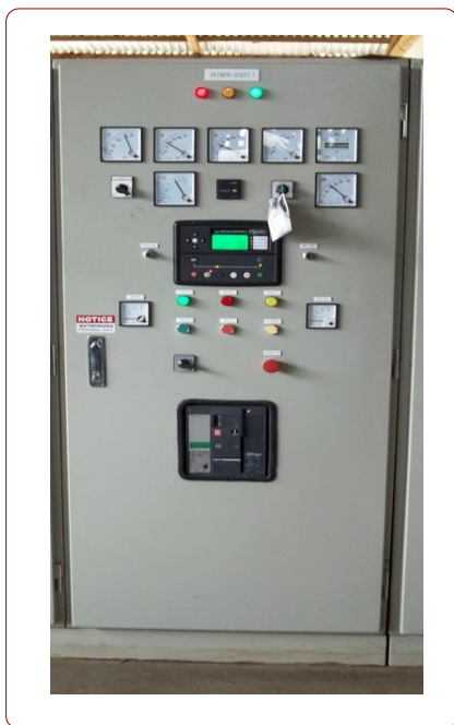
Generator Protection Panel
